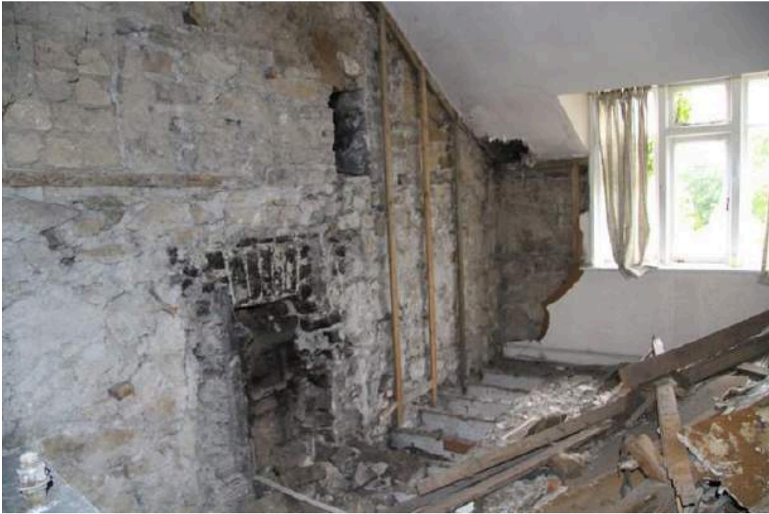
Plate No. 24. General View showing the current internal conditions at Frankfort Lodge. The entire structure is derelict and ruinous. The lodge was the result of extensive reconstruction of one of the former stable building, dating from ca. 1930.
