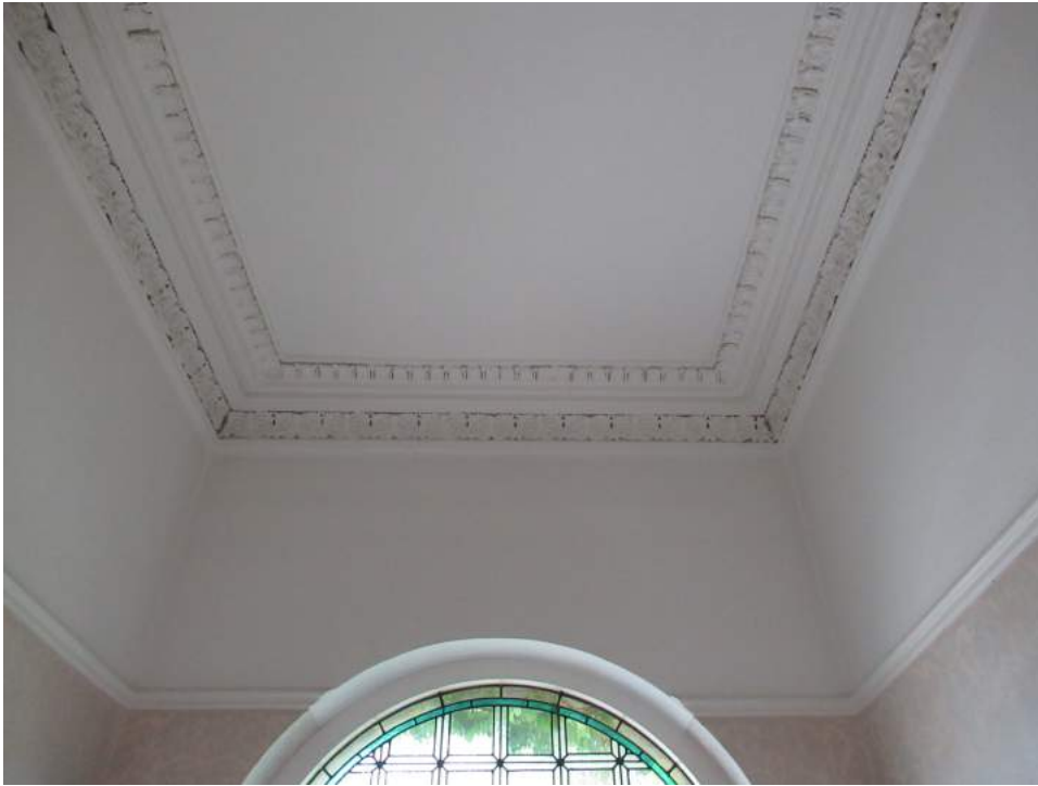
Plate No. 18. Detail view showing the ceiling in the entry hall in the northern half of the property. Close examination reveals that the wall at right, and the plaster coving above that wall, were later insertions into the original larger entry.
