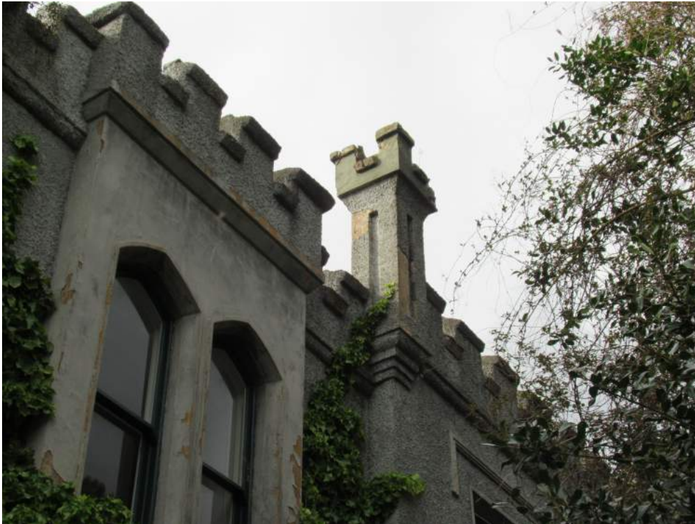
Plate No. 10. Detail view showing the mid-19 th century mock Tudor details on the east elevation. All of the patent cement renders and moulded features were covered with Portland cement dashing during the 20 th century. Some of the dash has fallen off revealing the 19 th century patent cement render beneath.
