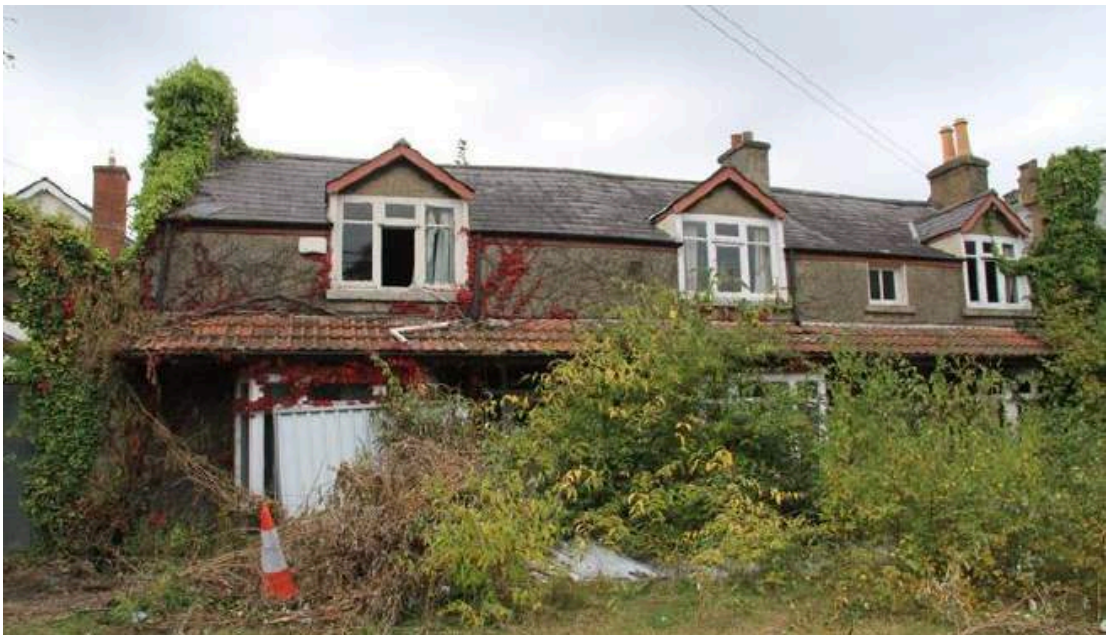
Plate No. 23. General View showing Frankfort Lodge, attached to the south end of Frankfort Castle.
