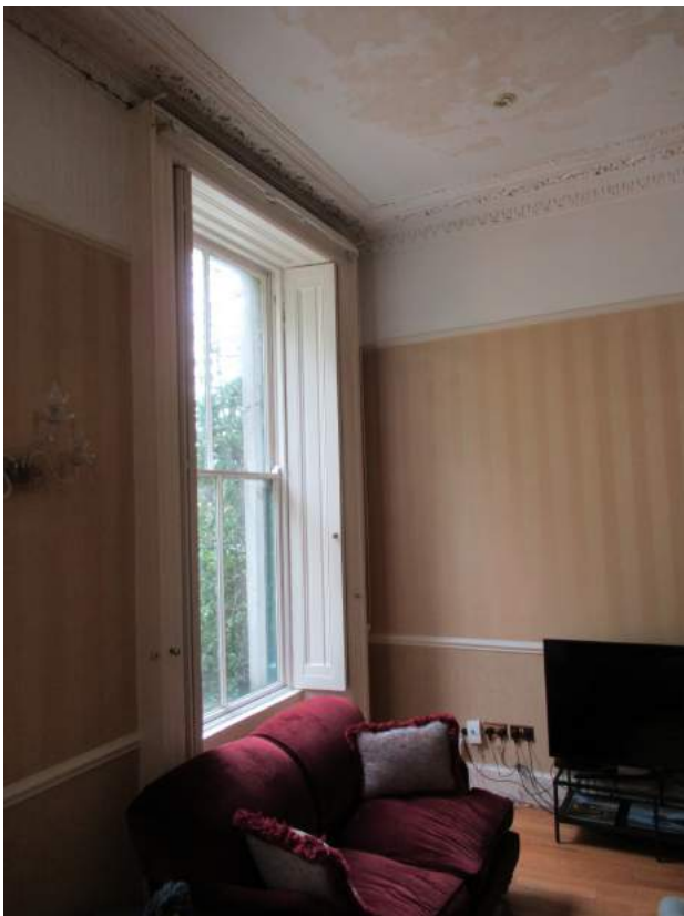
Plate No. 19. Detail view in the southern sitting room, showing the internal joinery and plasterwork dating from ca. 1860. Note the damage to the ceiling from leaking bathroom plumbing.
