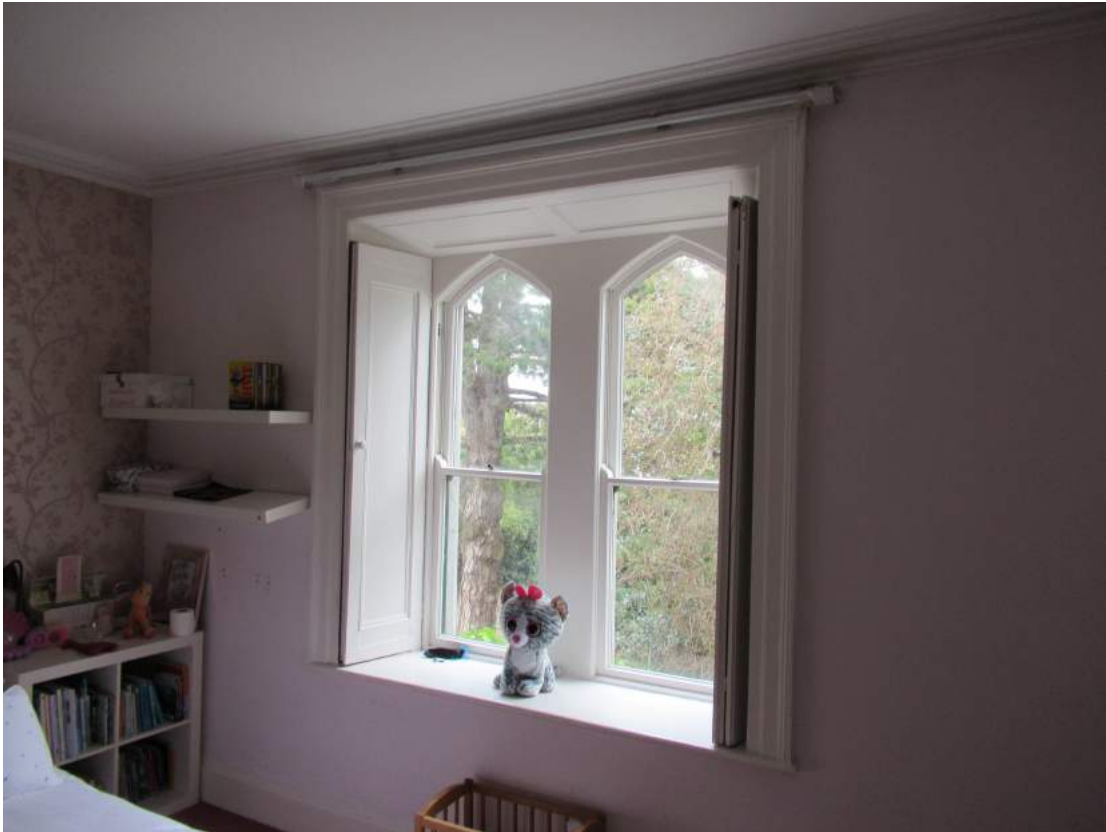
Plate No. 22. Detail internal view showing the internal window joinery in the first floor roof over the original entrance.
