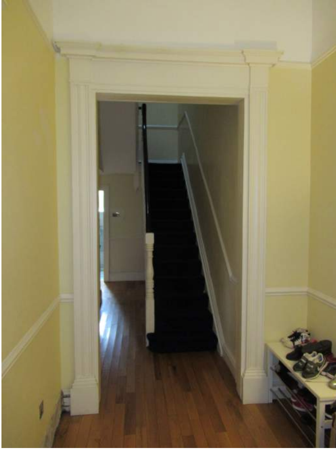
Plate No. 16. Detail view showing the stairwell in the southern half of the structure. This narrow stair likely dates to ca. 1930 when the original house was subdivided.
