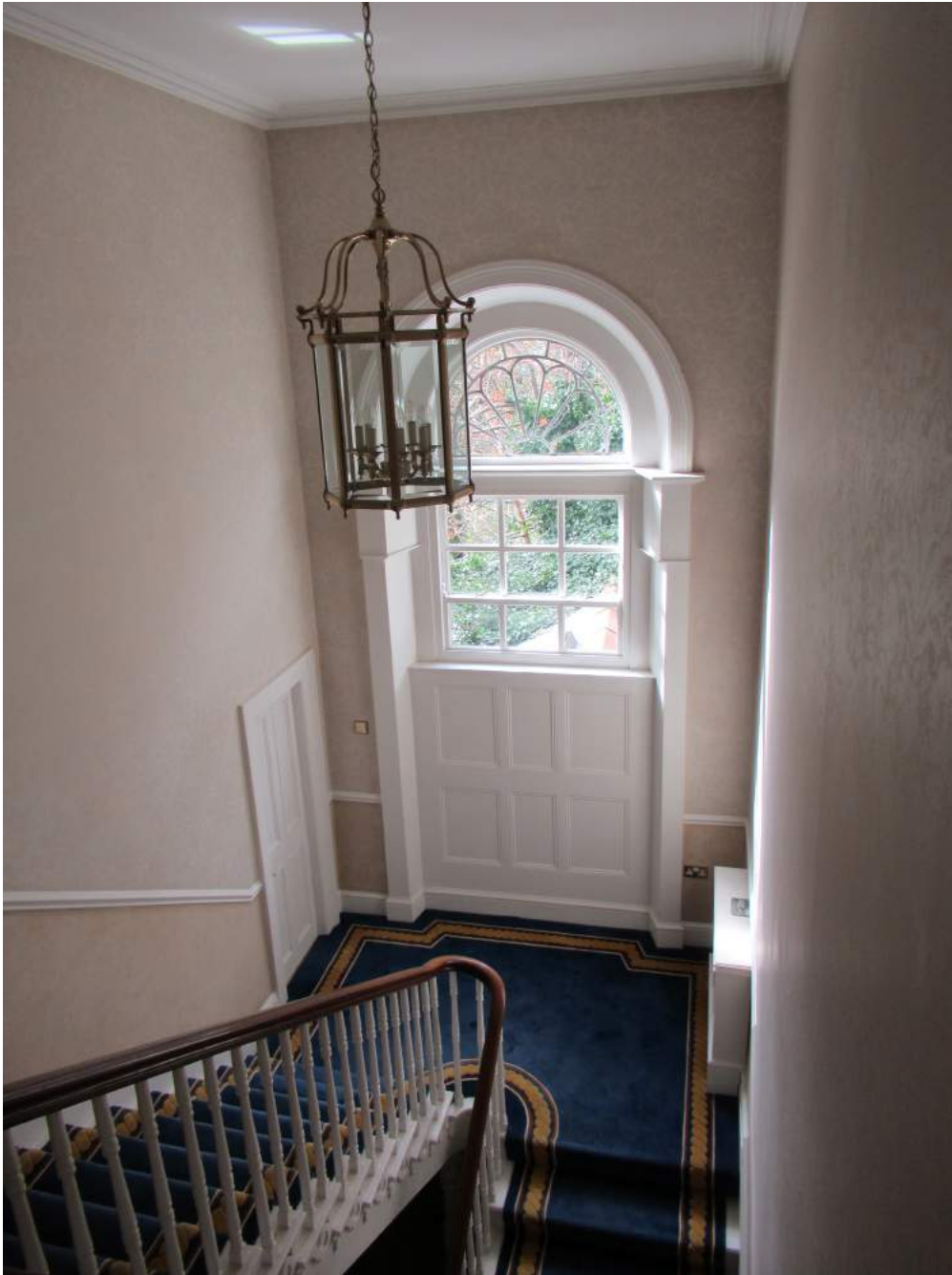
Plate No. 15. Detail view showing the stair landing in the northern half of the former Frankfort Castle. It is likely that the arched window originally extended nearly to the landing floor, but was partially blocked by the double pitch roof over an early 20 th century extension to the rear.
