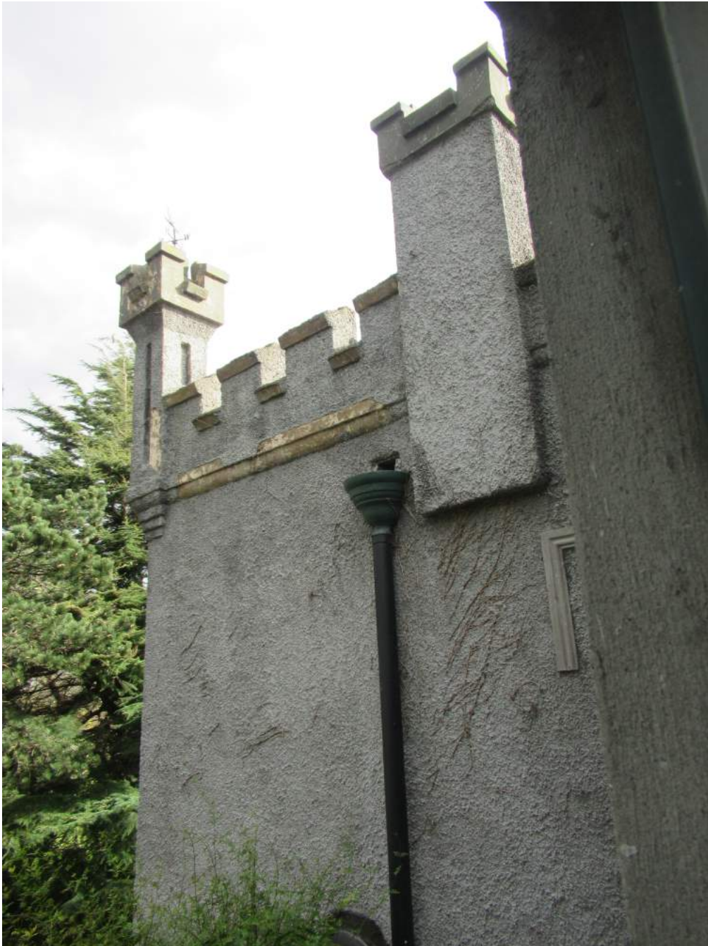
Plate No. 12. Detail view showing the north elevation of the original house, with the 20 th century extension at the right. Note the original patent cement moulded string course below the battlements, exposed by the failed cementitious dashed render. It appears that the earlier brown patent cement render had been finished with a yellowish finish coat.
